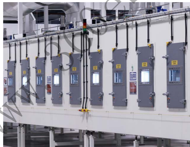
Electrode drying (one of the most energy intensive stages of the battery manufacturing process) at UKBIC
